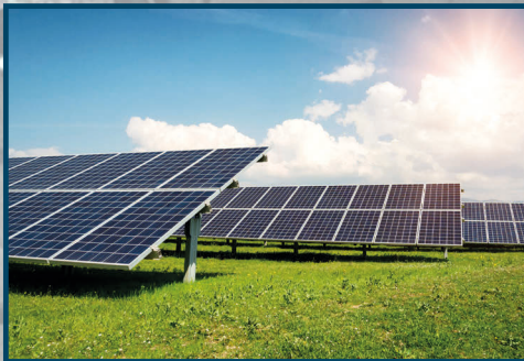
Pannelli solari / Solar panels
